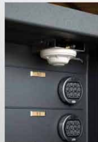
Thermal sensors and door contact
